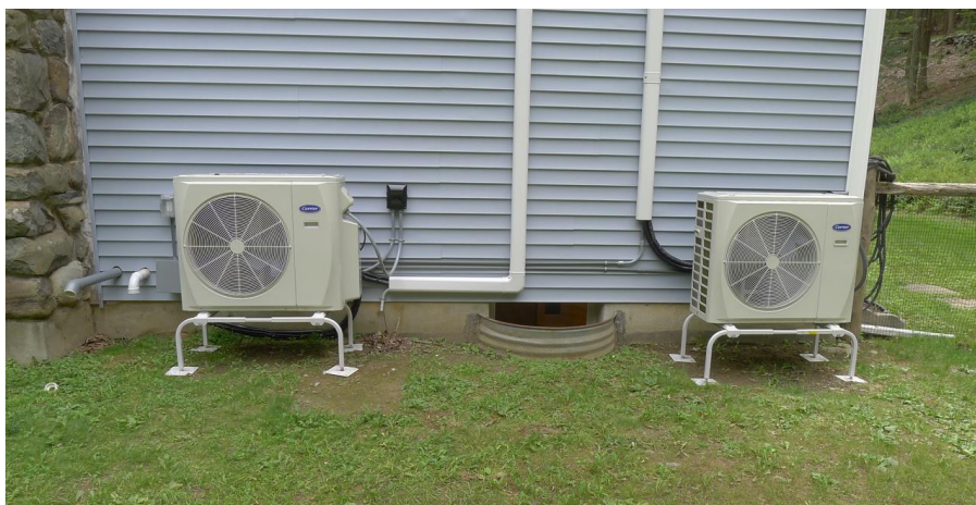
Figure 26: Air Source Heat Pump System Installed at a Central Hudson Customer Residence
