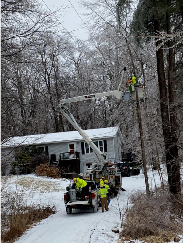
Crews work to restore service to a home in Salt Point, Dutchess County on Friday.
