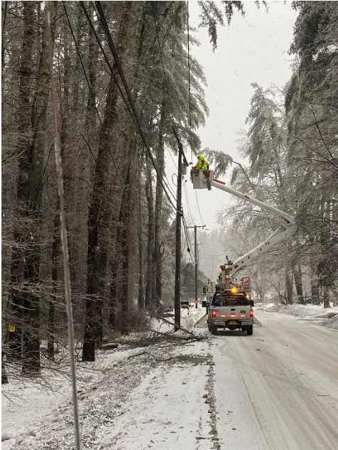
Central Hudson Crews work to repair a damage location in Woodstock, Ulster County.
