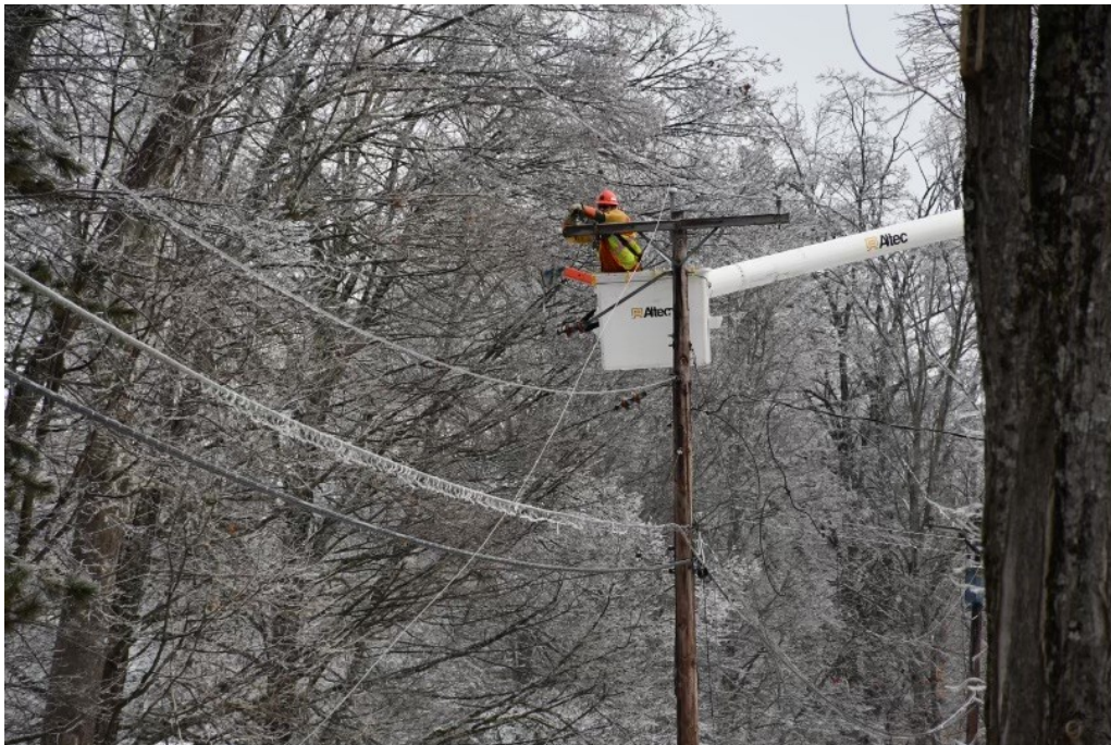
Crews work to repair damage on Berme Road in Marletown, Ulster County on Monday.
